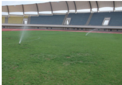
Irrigation system with poor overlapping of sprinklers
